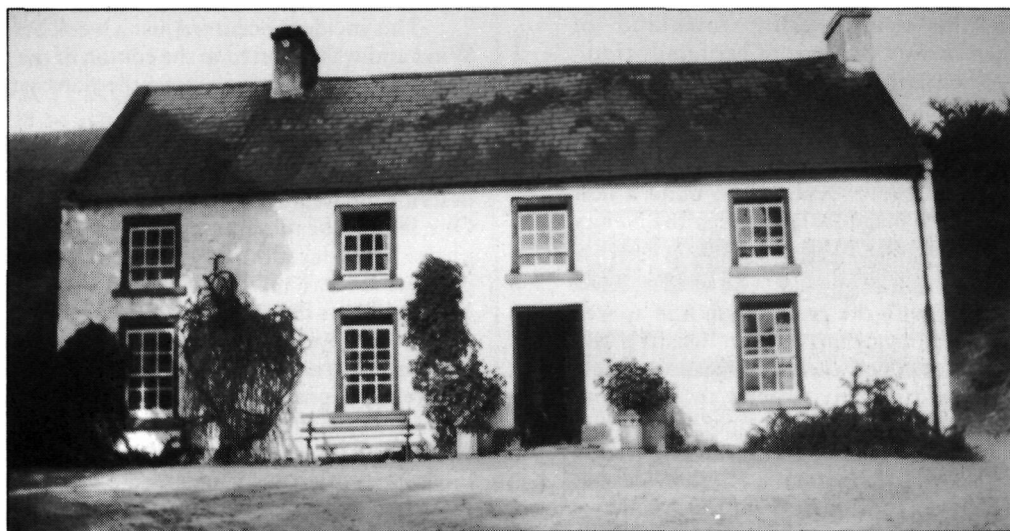
Prospect Hill, Latt, Jerrettspass. A stone dislodged from the chimney broke a hole in the front door.
